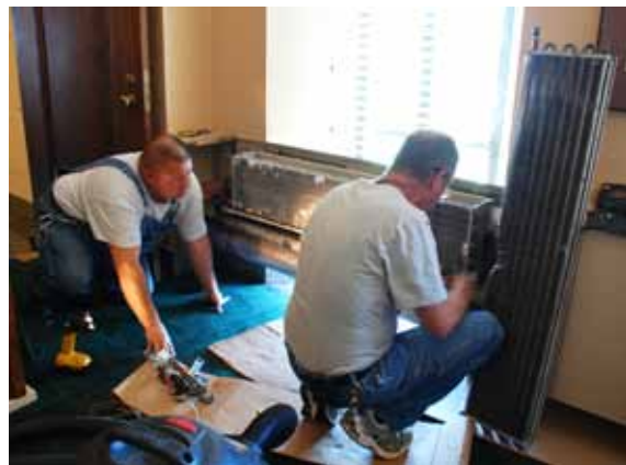
Above, shop staff put the finishing touches on a newly installed induction unit. The unit leaning on the right could not be repaired.
