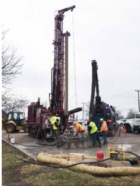
Above: Test wells drilled on the wellfield site in March allowed engineers to study the subsoil structure and plan for the most efficient configuration of the geothermal wells.
