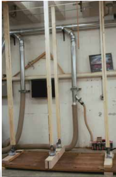
To apply gradual pressure on the warped desk top staff devised a press in the back of the shop. Left, using two by four boards, jacks, and the shop ceiling, the desk top was gradually flattened using the shop itself as a tool.
