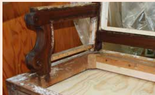
Above, staff repairs to the chairs included filling in the previously removed bottom support in the back of the chair seat and filling holes left by tacks and staples. The back structure required the staff to reinforce the wooden insert which holds the webbing. They screwed poplar to the frame, a longer lasting solution than the previous nailed on pine.
