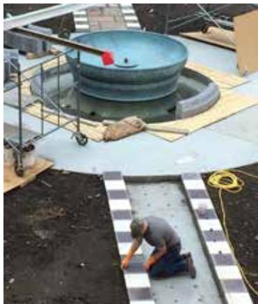
Left, Erv Wemhoff with Cornhusker Tile set the marble pavers in the walks during the 2017 fountain installation. Wemhoff returned to install the glass tile in the fountain bowls.
