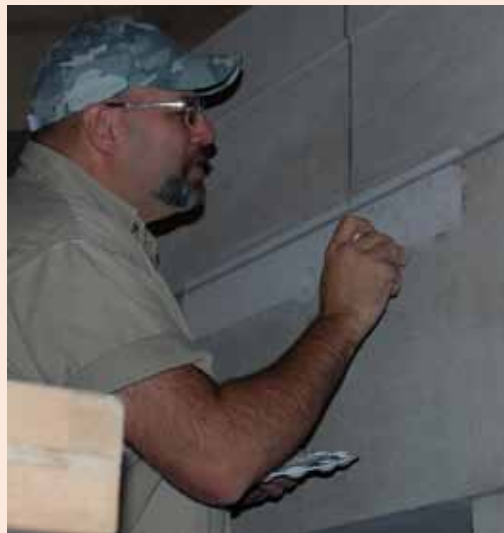
Once the mortar patch was dry, OCC staff blended the edges and created mortar joint lines in the patched area.
