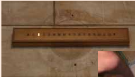
Behind the lighted bar floor indicator, installed in the 1950's, the shadow of the original circular elevator floor indicator dial is visible, left.
