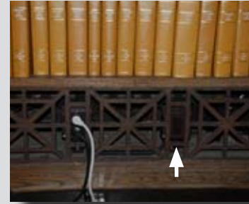
Two new outlets were located in bookshelves and are unnoticed except when in use, left.
