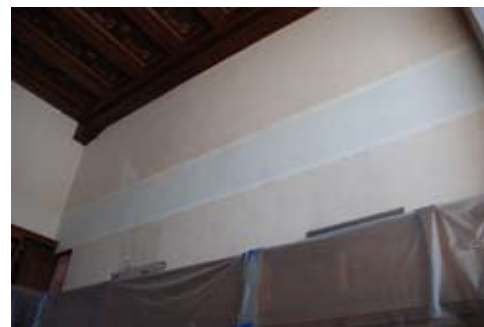
Plaster repair, above, covering the stabilized wall support beam will be monitored to gauge success of repair.
