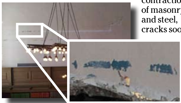
Damaged plaster reveals a hint of color and what might be a decorative finish.
