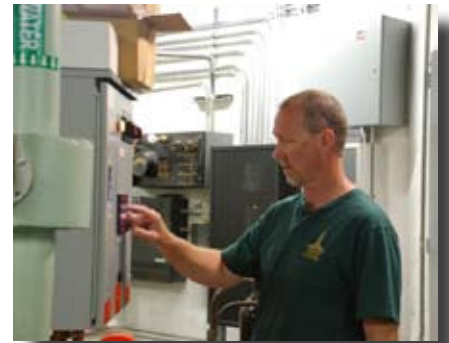
Michael Jordan, Maintenance Supervisor, checks an alarm on the tower's domestic cold water booster pumps.
