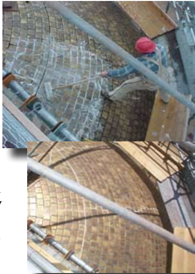
Once contractors completed the gentle cleaning and grouting, the Capitol's dome was ready to shine.
